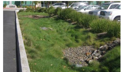
Figure 50. On-site storm water capture.
