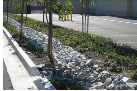
Figure 17. On-site stormwater capture system.
