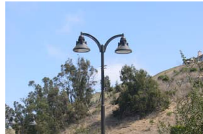
Figure 12. Hooded light fixture directs light downward.
