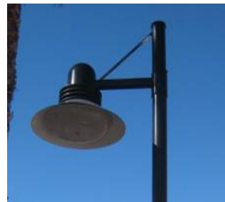
Figure 46. Pole mounted light.
