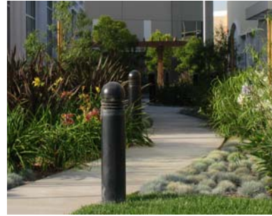
Figure 45. Bollard lighting along pedestrian walkway.
