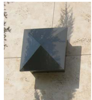
Figure 14. Decorative light fixtures.
