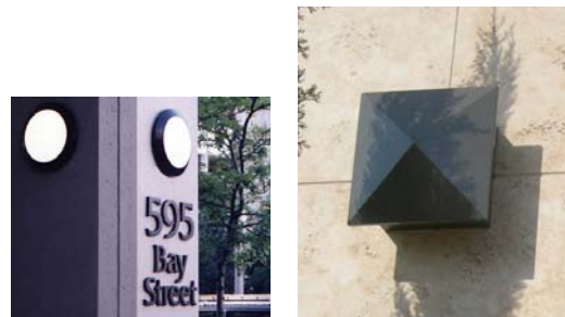
Figure 47. Decorative light fixtures.
