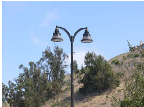
Figure 44. Hooded light fixture directs light downward.
