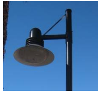
Figure 46. Pole mounted light.
