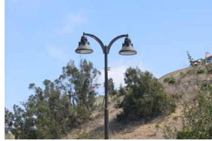
Figure 44. Hooded light fixture directs light downward.
