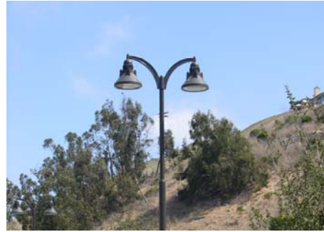
Figure 44. Hooded light fixture directs light downward.
