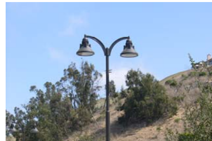
Figure 12. Hooded light fixture directs light downward.
