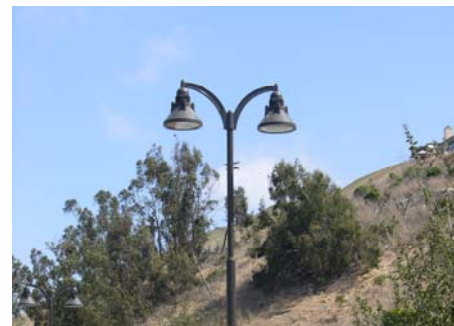
Figure 44. Hooded light fixture directs light downward.
