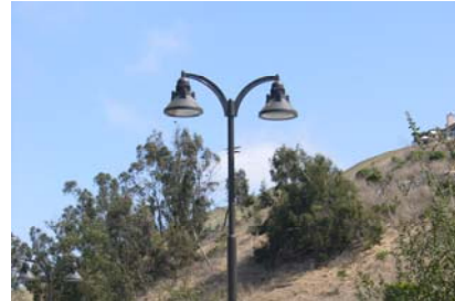
Figure 12. Hooded light fixture directs light downward.
