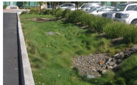
Figure 50. On-site storm water capture.
