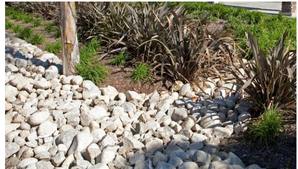
Figure 79. On-site stormwater capture system.
