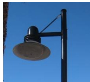
Figure 46. Pole mounted light.
