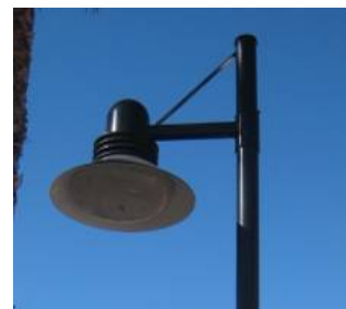
Figure 46. Pole mounted light.
