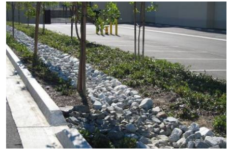
Figure 17. On-site stormwater capture system.
