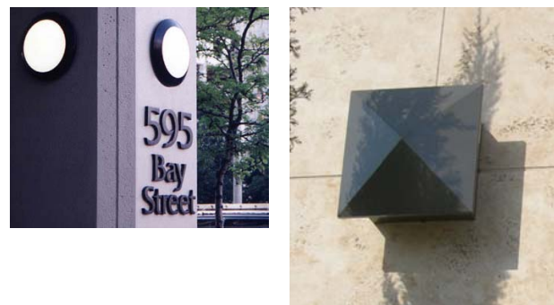
Figure 14. Decorative light fixtures.
