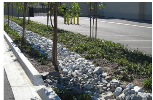
Figure 17. On-site storm water capture system.
