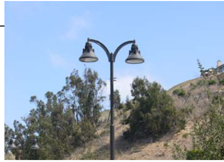
Figure 44. Hooded light fixture directs light downward.
