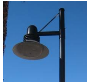
Figure 46. Pole mounted light.
