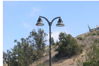
Figure 12. Hooded light fixture directs light downward.
