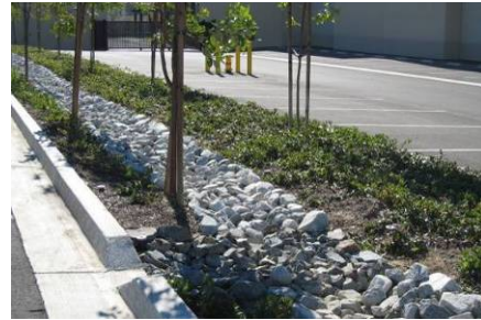
Figure 17. On-site stormwater capture system.
