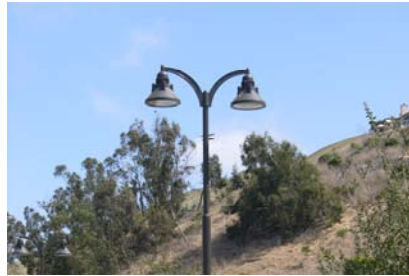
Figure 12. Hooded light fixture directs light downward.
