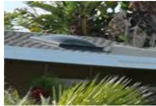
Inappropriate: Domed Skylight
