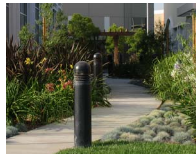
Figure 45. Bollard lighting along pedestrian walkway.
