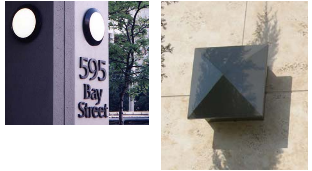
Figure 14. Decorative light fixtures.
