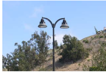
Figure 44. Hooded light fixture directs light downward.
